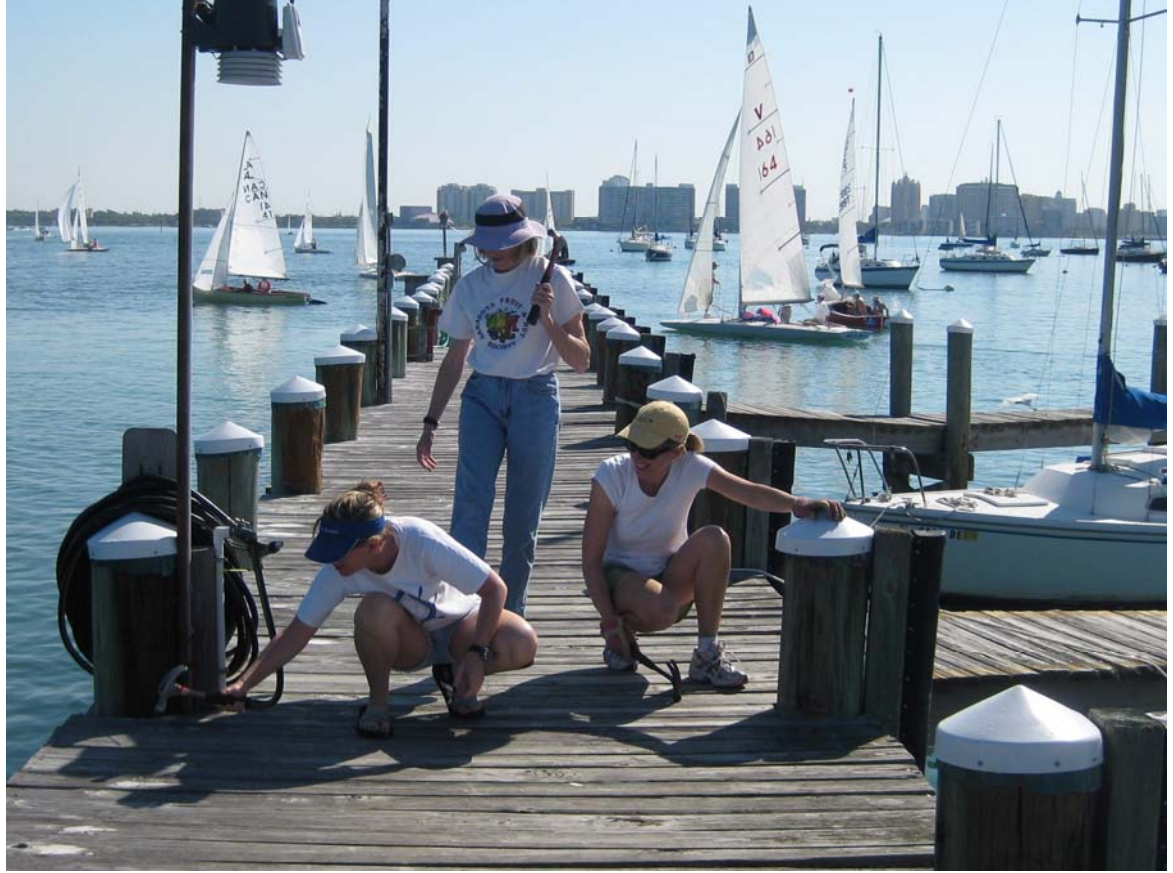
Julie Burnett, Suzy Conover and Diane Banyard work on dock repairs as the Mid-Winters fleet sails out. Photo by Rachel Harvey
